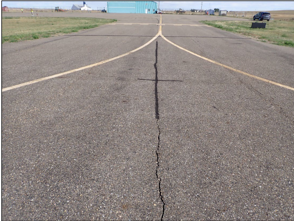
TW-01-01: L&T Cracking
