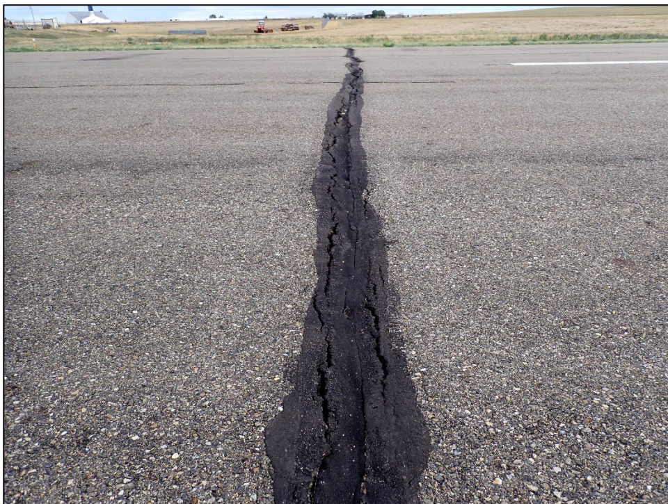
RW11-11-26: L&T Cracking
