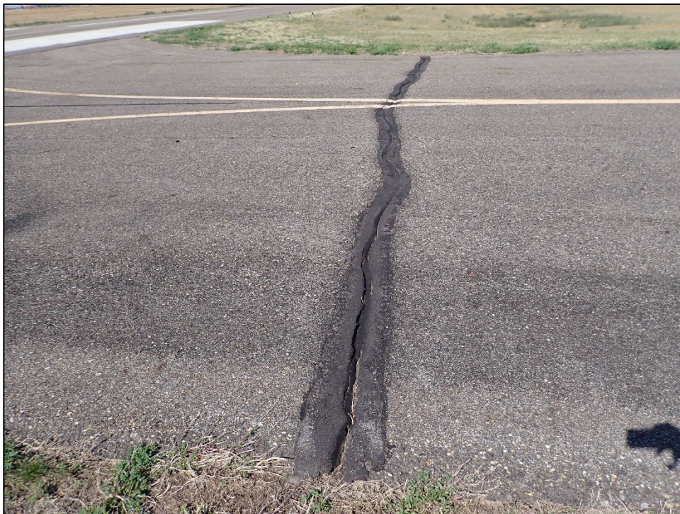
TW-02-01: L&T Cracking
